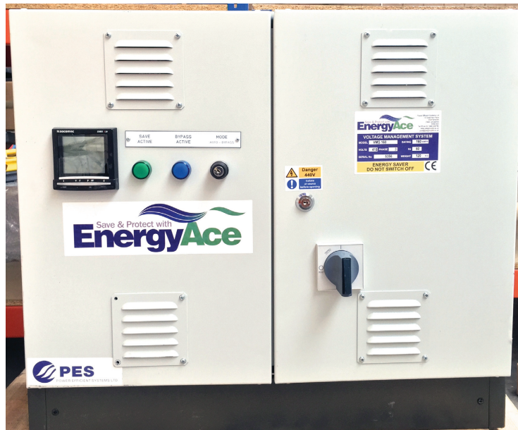
With so many variables on many sites power quality is now more of an issue than ever before
